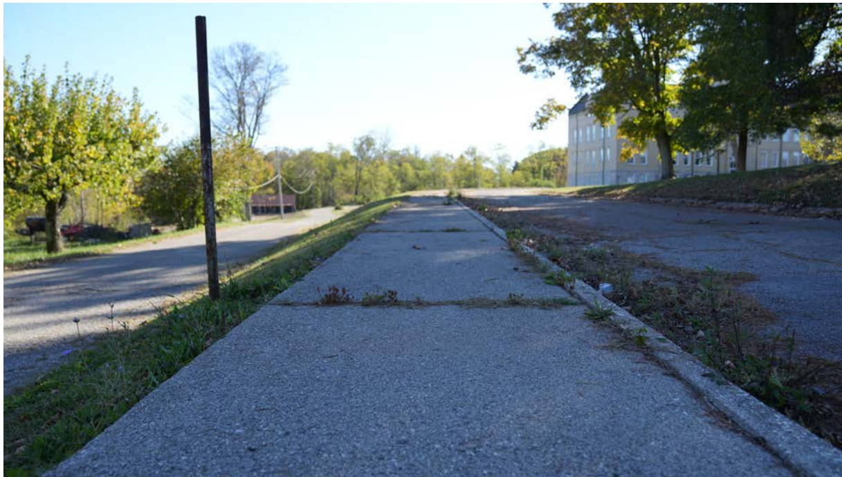
Challenges due to gaps in the overall sidewalk network remain.
